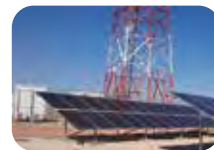
Saudi Arabia-Telecom Station
